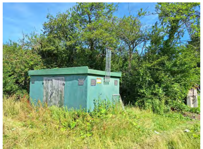
Gas installation in north east corner of site.
