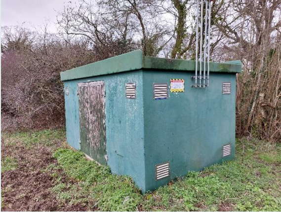
The Gas Installation Adjacent to the Site Entrance
