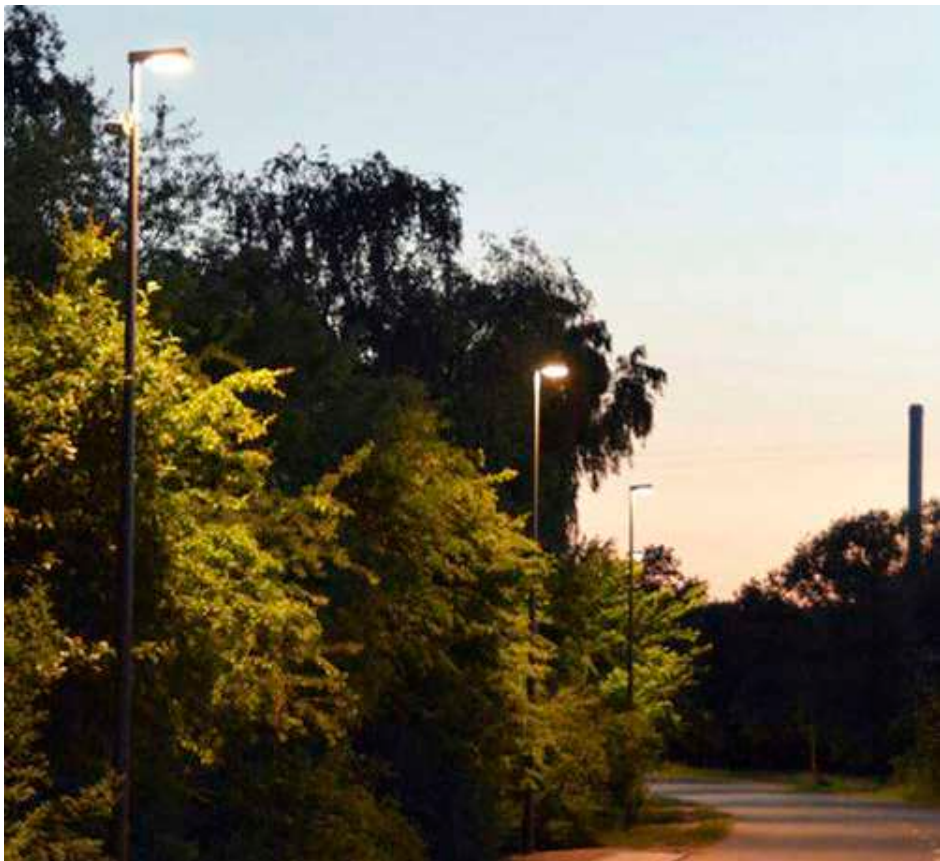
Column lighting to highways
