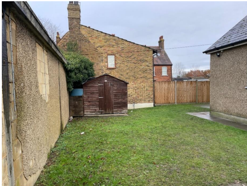
Existing flank wall of No.2 Farm Cottages and building to be demolished on the left
