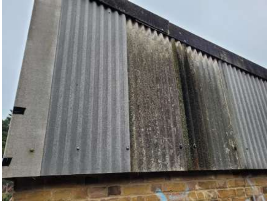
Photo 6 – View of southern end of storage barn, showing suspected ACM.
