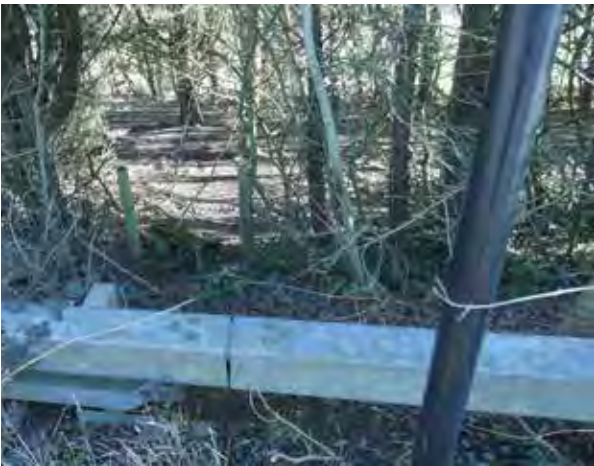
AW276, poor access and condition.
