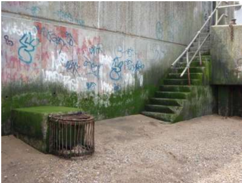
SW outfall into the Thames from Pier Road.
