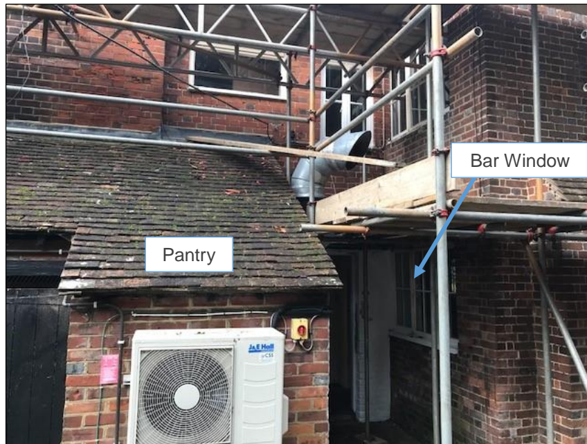
Photograph showing the bar area where music may be performed and the adjacent pantry
