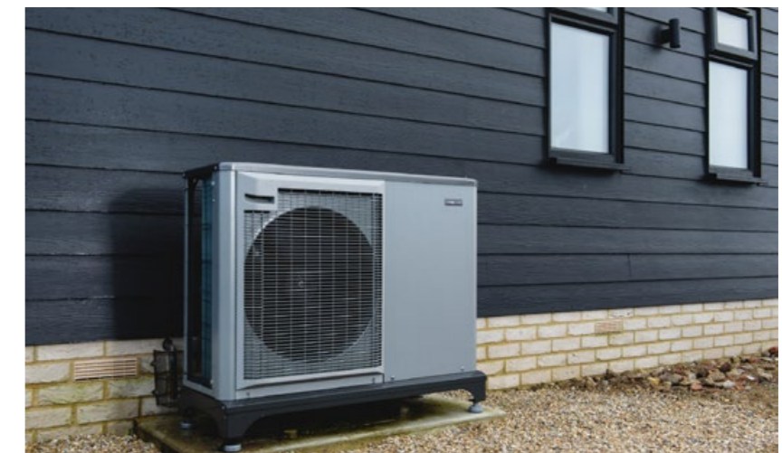
Air source heating unit
