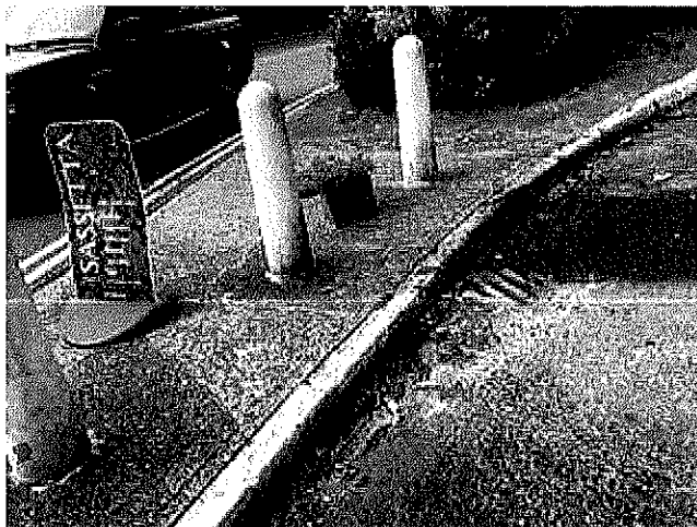
Figure 3: Blocked gully could compromise pedestrian safety.
