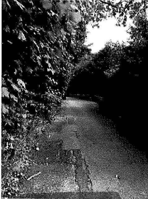
Figure 2: Overgrown vegetation could compromise pedestrian safety.
